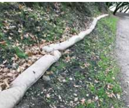
Straw wattles placed to slow and dissipate water, with rolls overlapping. Photo by Rich Casale
